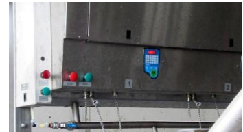
Auto-milker control panel
